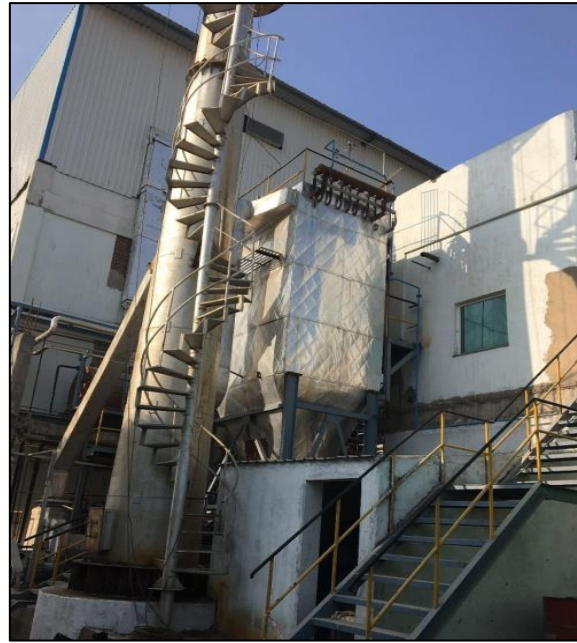
Bag filter attached with boiler stack
