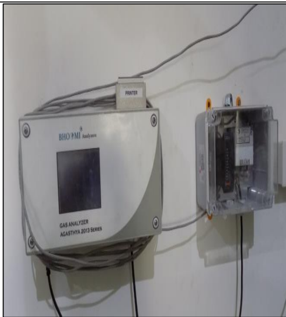
Boiler SPM Monitoring Panel
