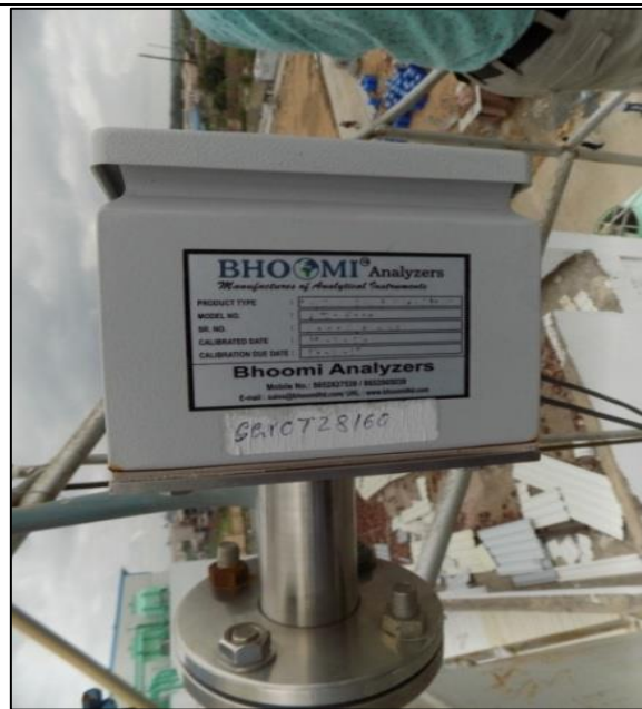
Boiler Stack Monitoring Sensor
