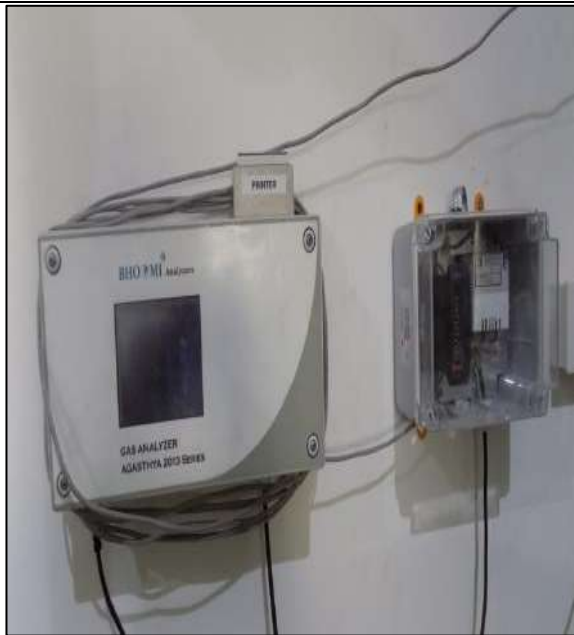
Boiler SPM Monitoring Panel
