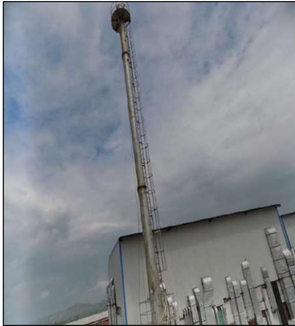
Adequate height provided to boiler stack
