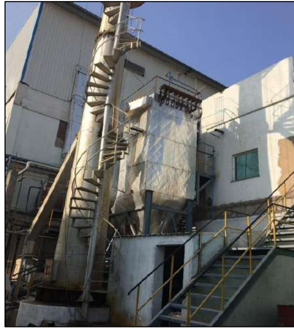
Bag filter attached with boiler stack
